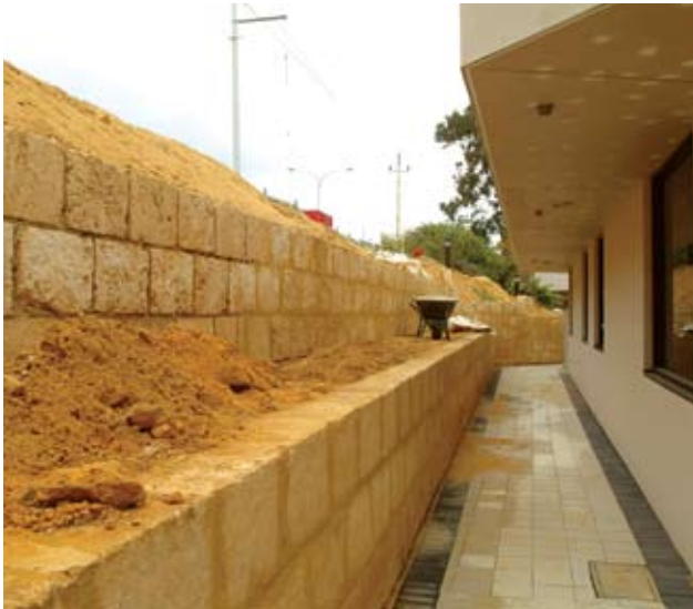
Closeness of retaining wall to building causes landscaping challenges.
