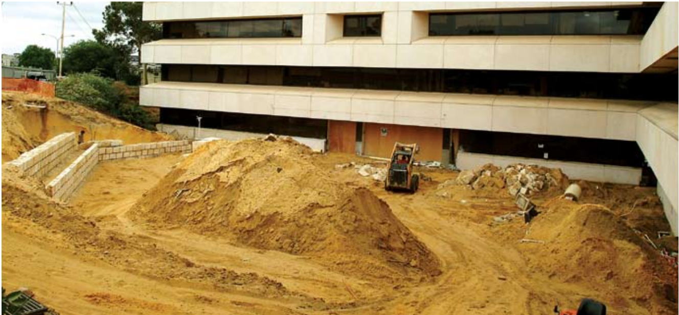
External view of the site looking south – note the steep bank and retaining wall. With a major arterial road to the east.
