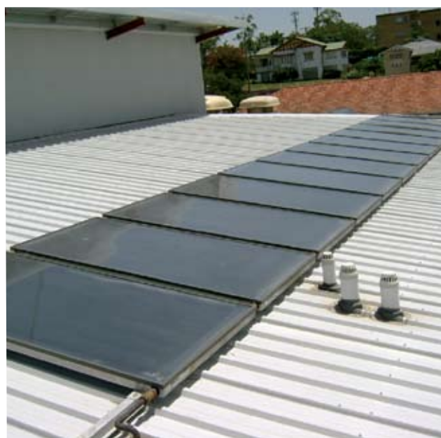
Solar heaters as installed
