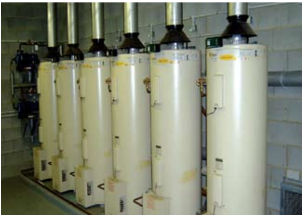
Existing gas hot water cylinders
