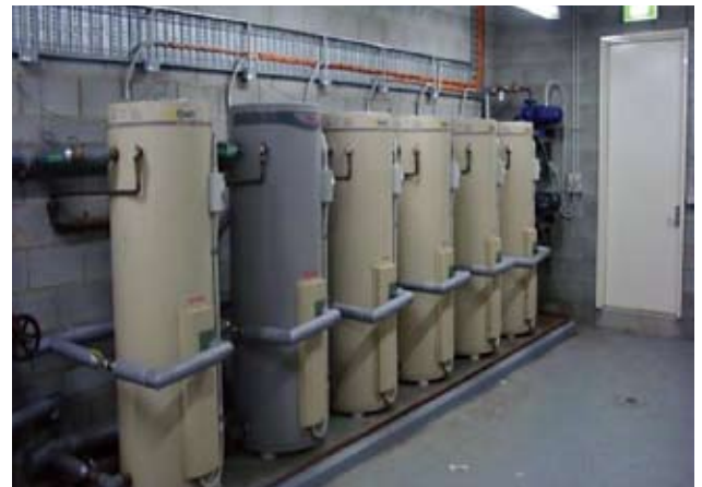
Modified electric hot water cylinders
